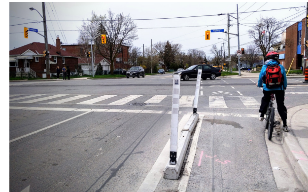
Upgrading existing bicycle lanes or cycle tracks for safety and comfort by adding physical protection such as pre-cast curbs, planters or poured-in-place concrete medians.
